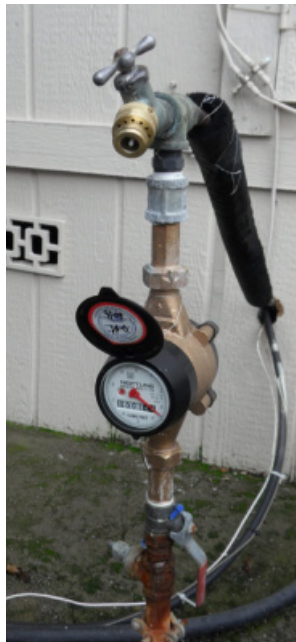
Submeter at a mobile home park
