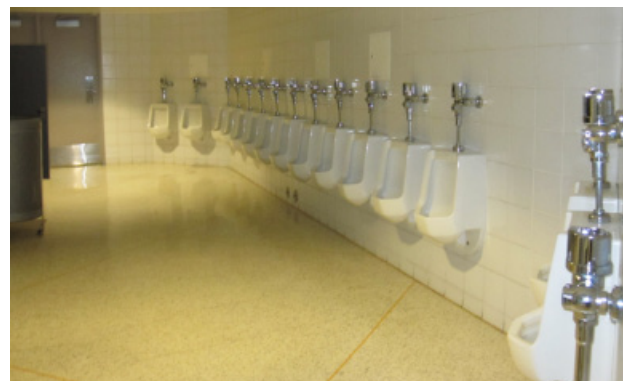
Urinals at HP Pavilion
