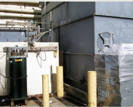
Example of cooling tower system
