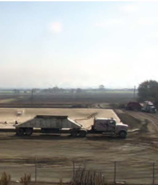
The new 3 million gallons-per-day grant-funded water reservoir in the SCRWA treatment plant
