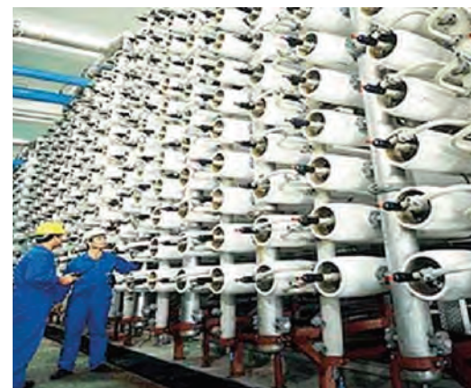
Example of a membrane treatment facility for desalination.
