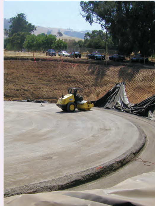
The Zone Three Reservoir is under construction and will have a storage capacity of 55 million gallons.
