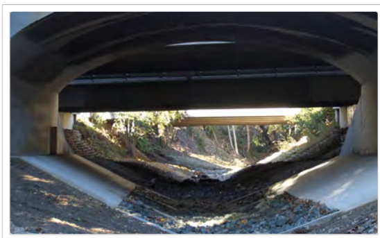
Construction of a fish passage channel in Stevens Creek under the Evelyn Avenue Bridge.
