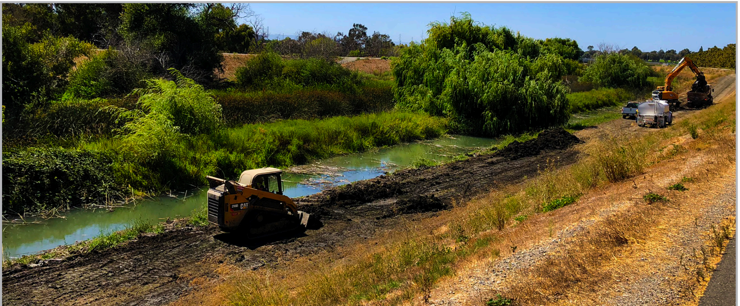
Valley Water maintenance work to remove sediment along the east bank of Guadalupe River, upstream of Tasman Drive.
