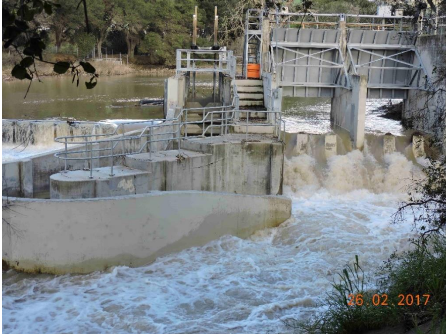
Photo 5. Metcalfe Pond radial gates and impassable (no flow) fish ladder on 26 February 2017.
