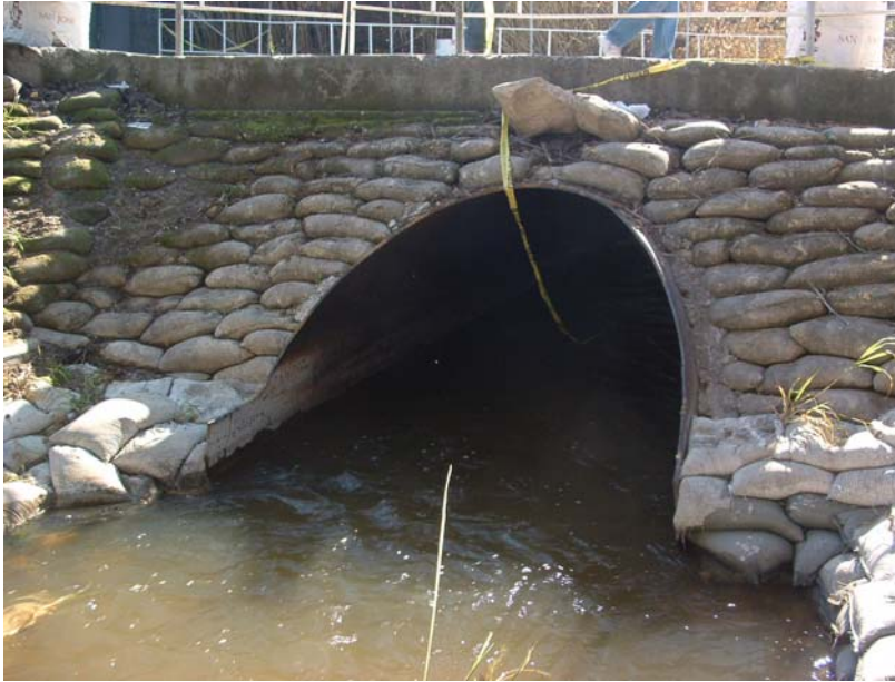
Figure 3. Entrance to the culvert located upstream of the confluence Coyote Creek in Upper Penitencia Creek .
