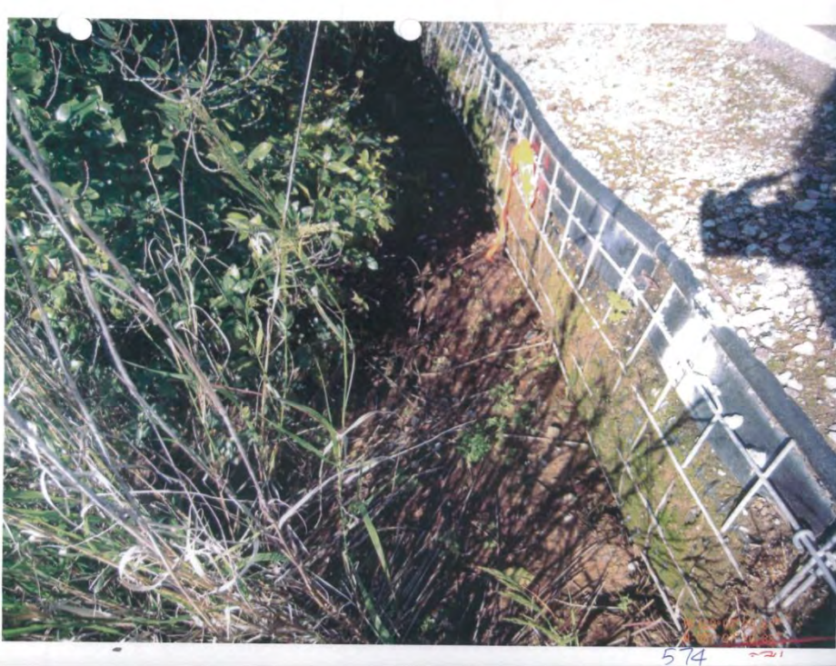
Hole with seepage at lift (SCVWD 574) – 12/27/2012
