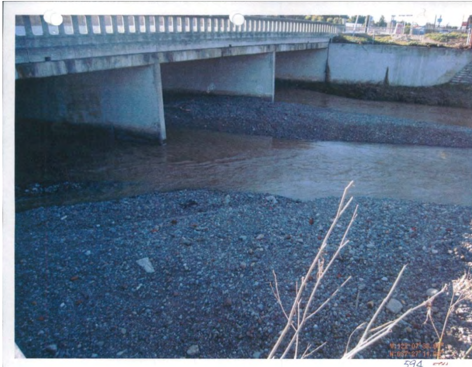
Sediment under (upstream) of Bayshore Road (SCVWD 594) – 12/27/2012
