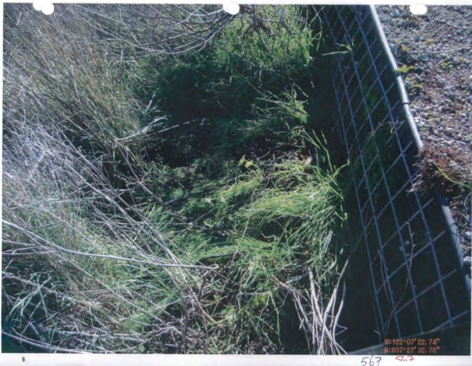
Minor void / seepage through lift (SCVWD 567) – 12/27/2012
