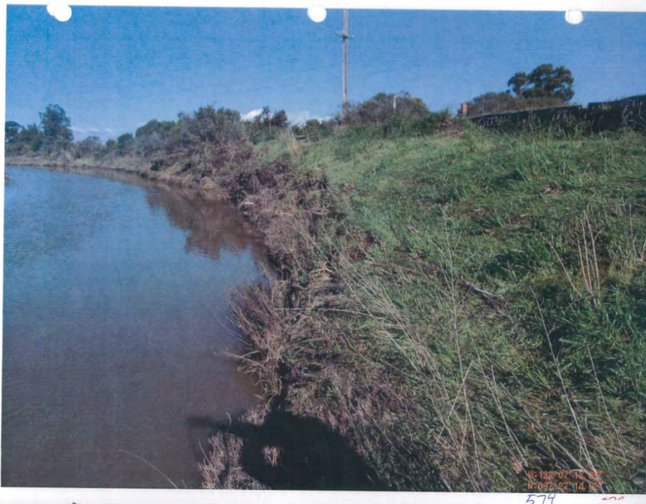
New sloughing inboard (SCVWD 579) – 12/27/2012
