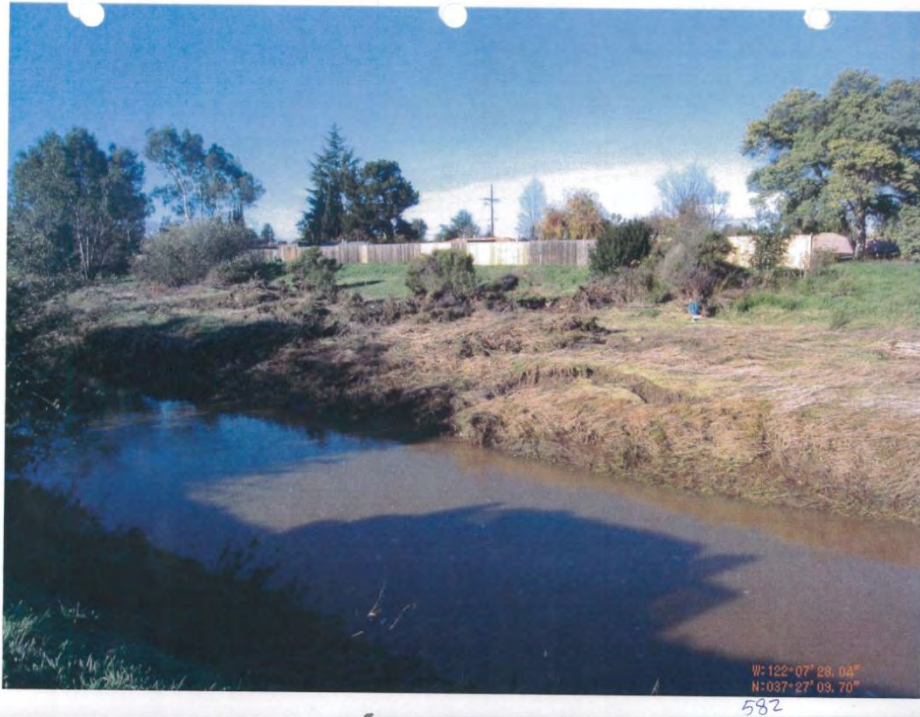
New sloughing located on the opposite bank (SCVWD 582) – 12/27/2012
