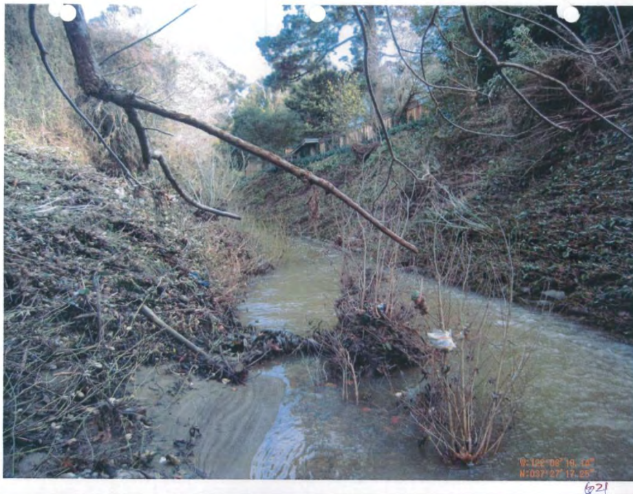
Narrowed channel due to sediment and vegetation (SCVWD 621) – 12/31/2012
