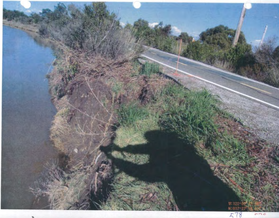
New sloughing inboard (SCVWD 578) – 12/27/2012
