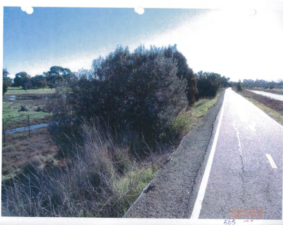
Woody growth – “no visual of levee” (SCVWD 565) – 12/27/2012
