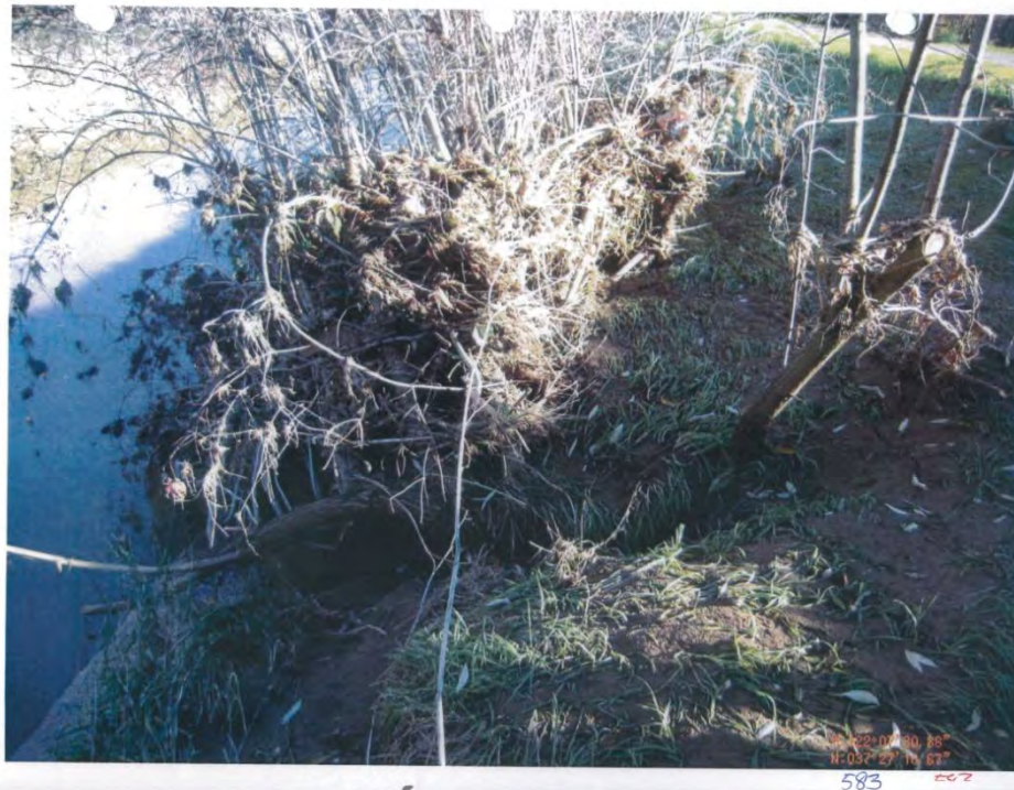
Minor rilling at the International School of the Peninsula inboard (SCVWD 583) – 12/27/2012
