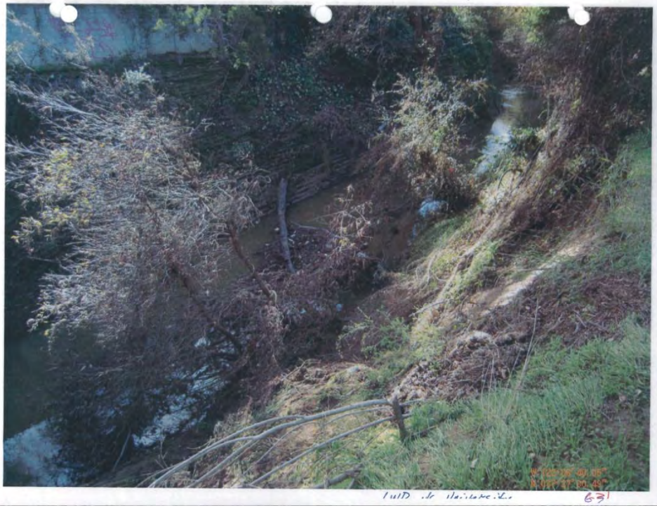
Minor blockage across from 1523 Woodland Avenue (SCVWD 631) – 12/31/2012
