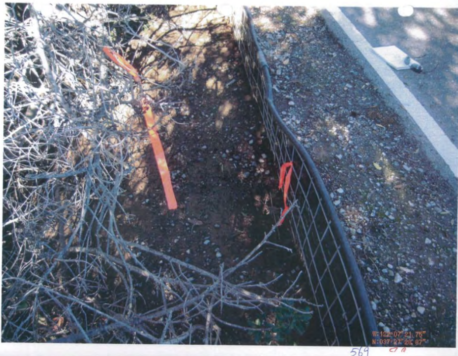
Rodent hole at lift – noted “seepage?” (SCVWD 569) – 12/27/2012
