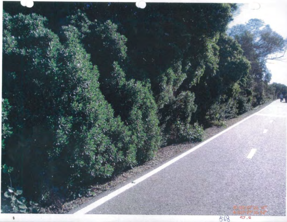
Woody growth on levee – no visual inspection (SCVWD 568) – 12/27/2012
