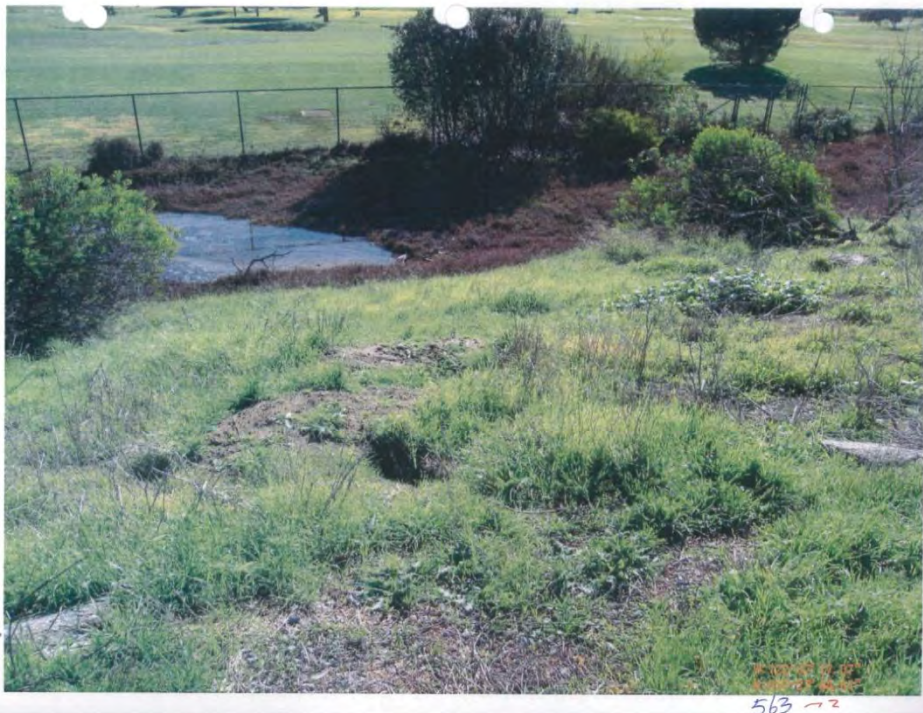
Rodent hole (Foreground) Standing water (Background) (SCVWD 563) – 12/27/2012
