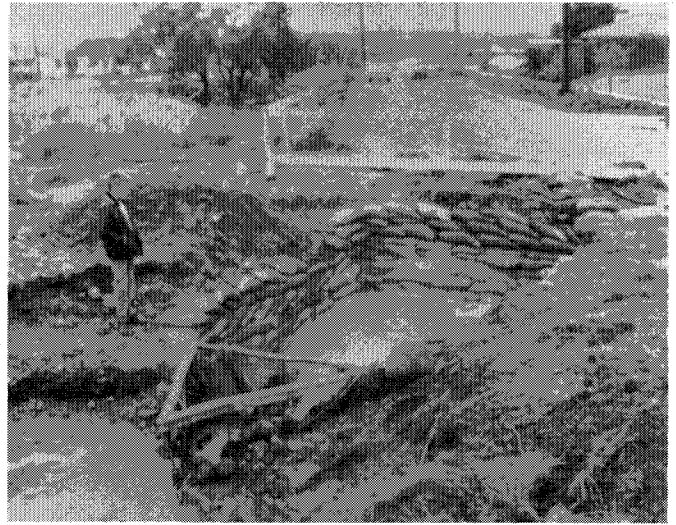
Crosley Ck intake after clamshell clean-out. Flow coming out of 1st manhole at car in distance.
