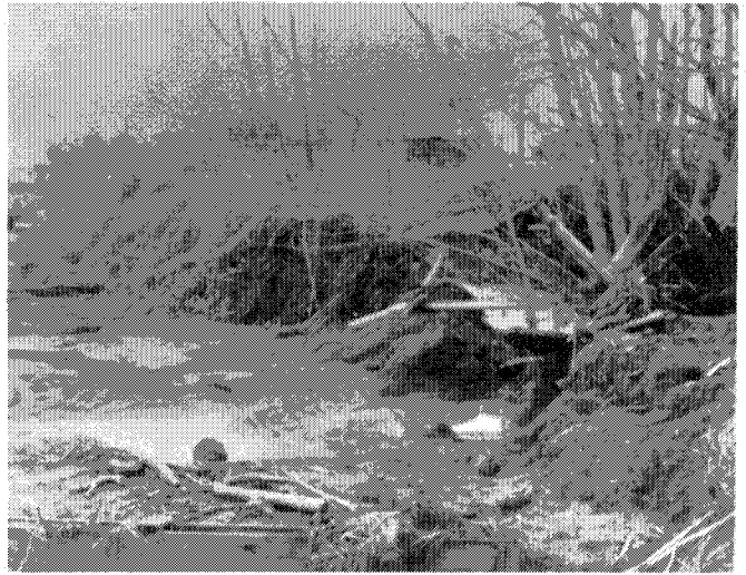
#22 Major breakout on Berryessa Creek left bank about 400 feet east of Morrill Rd.
