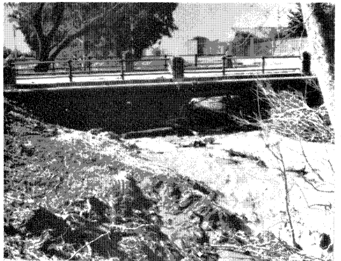
Looking downstream at the Noble Avenue Bridge over Penitencia Creek. Shadows obscure large amount of debris that is caught on bridge pier and abutments. High water topped this bridge at a depth of about 6 inches.
