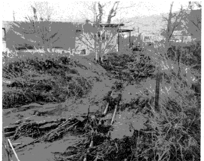
Breakout left bank Berryessa Ck. about 100 feet upstream of that shown in #22 and 23. Irrigation flume shown installed thru levee
