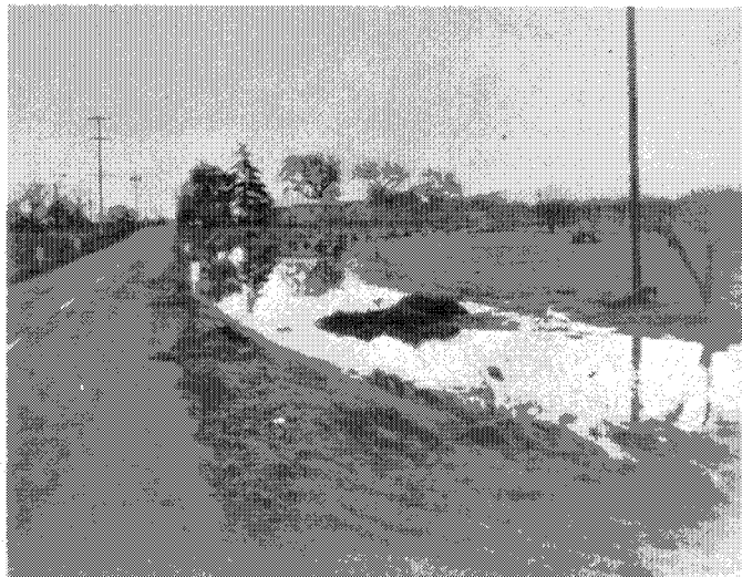
Sharp bend in Little Llagas Creek 3400 feet south of Middle Avenue next to Sycamore Avenue. Debris on road and in trees.
