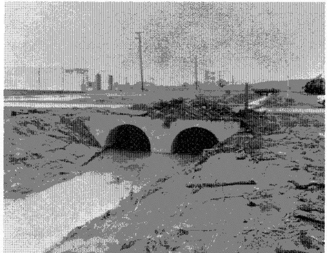
Berryessa Creek at Landess Avenue looking downstream. Trash on headwall was piled there by maintenance crew. Water topped both banks and spread across Landess Avenue about 6 inches deep.
