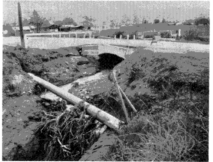
Looking upstream at the Cropley Rd. culvert over Berryessa Creek showing serious erosion under San Jose Water Works' main and collapse of the culvert extension on the northerly side of Cropley Road.
