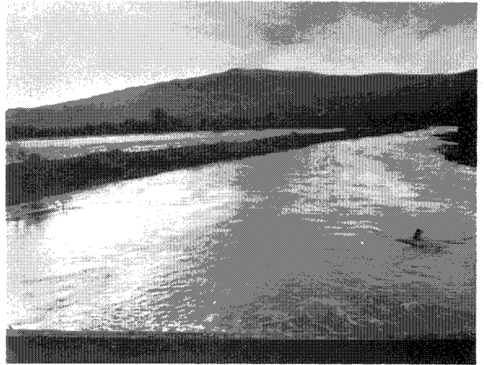
Carnadero Creek at farm bridge near Pajaro River. Note ponding out- side of left levee.
